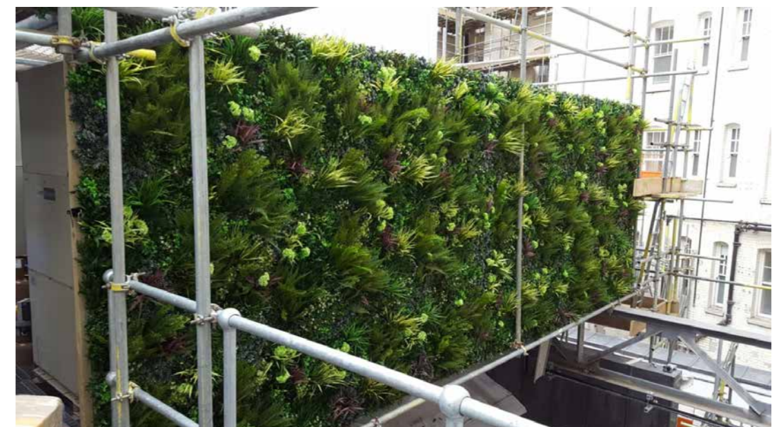
Completed project dressed with Delicate White Colour Box prior to install due to complicated access to the wall
